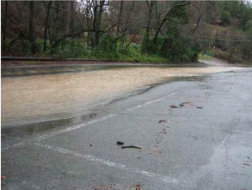
Photograph 6: Flooding along Smith Flat Road
